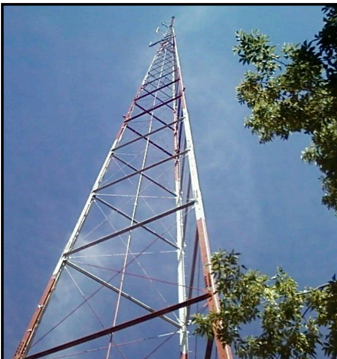
The 350-foot tall tower that will be used to transmit GSCR programming to the Jackson area.
